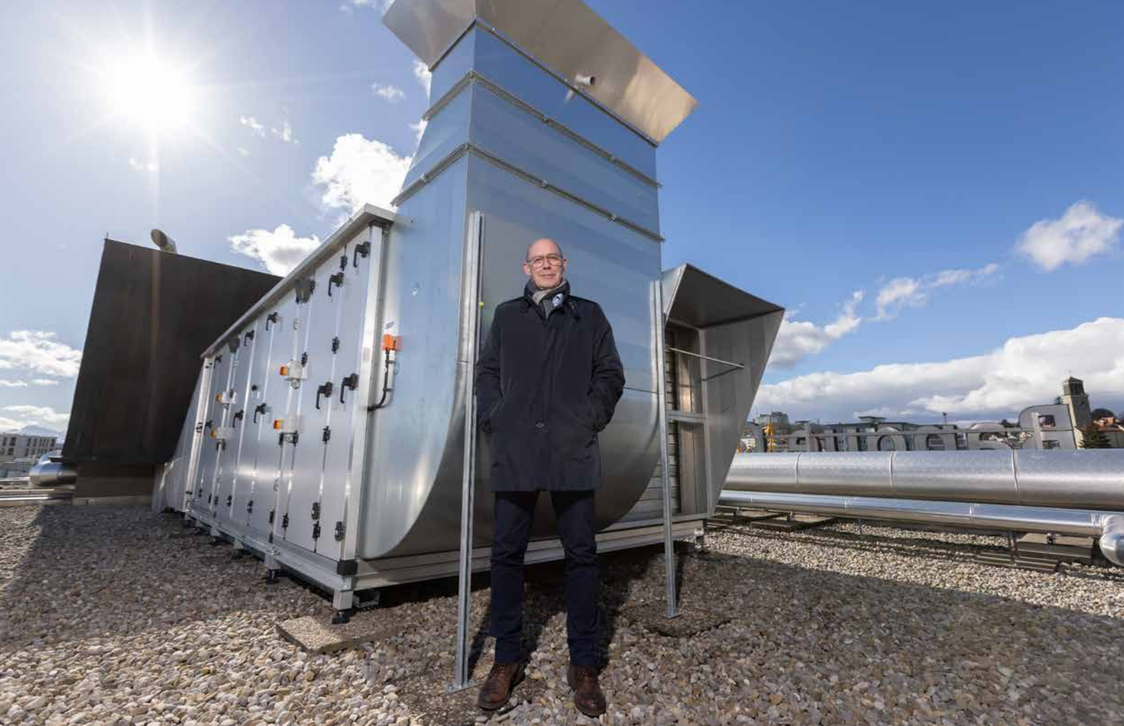
Patrick Neuhaus, Head of Real Estate and Logistics, in front of the monobloc at the top of the headquarters
